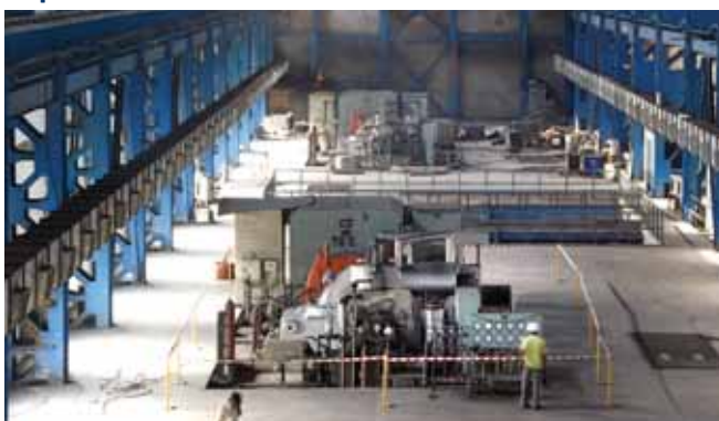
Captive Power Plant
