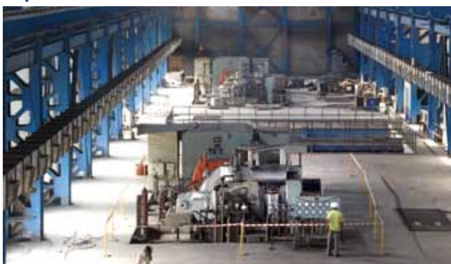
Captive Power Plant
